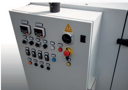
Control panel and security system integrated in the electrical panel. Operating mode AUTO / MAN with the possibility of managing the extrusion line speed signal.
